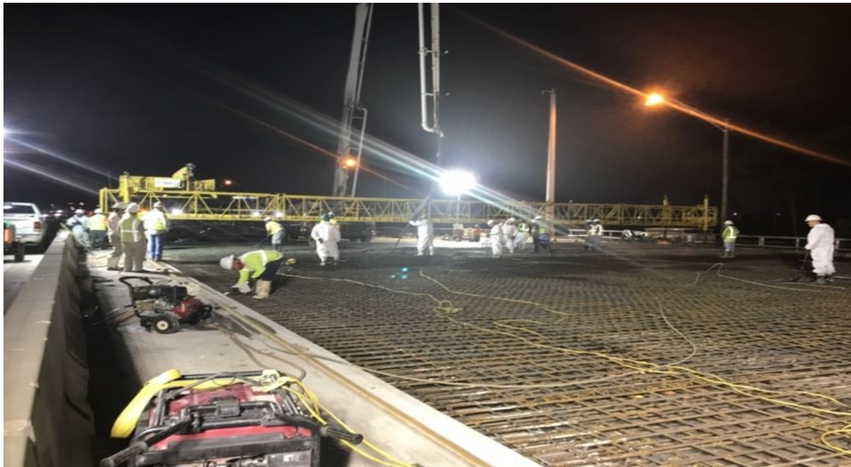
Final concrete deck pour operations along I-95 southbound for the complete reconstruction of the Hillsboro Canal bridge
